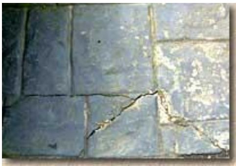
Cracking and Flaking of PIC
